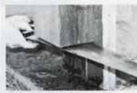
10" rotted bottoms of these load-bearing columns...
