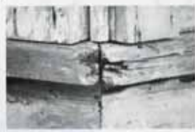
This rotted - and irreplaceable - woodwork...
